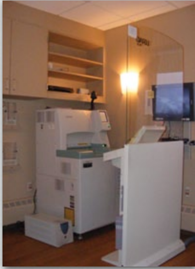
Mammography CR (computerized radiography) equipment and a mammography control console in one of the recently expanded breast-imaging services suites.
